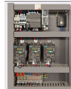
SIEMENS Electrical Cabinet
